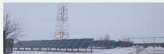
Semizbay-U's PV power plant
