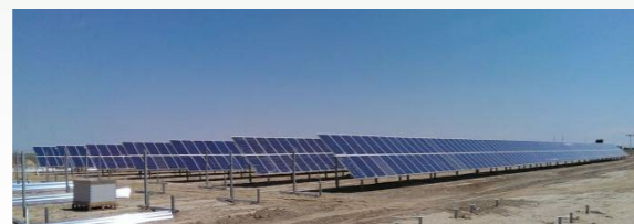
Ortalyk's PV power plant
