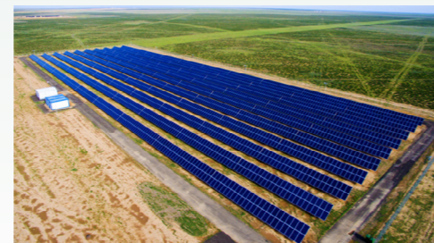
Photovoltaic Power Station
